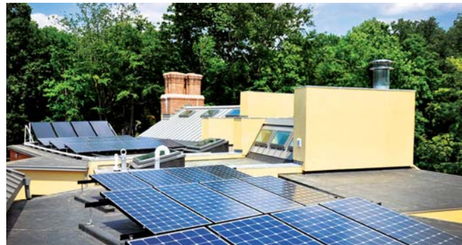
The metal roof features an array of 10-kilowatt solar panels. Excess hot water generated by solar energy is dumped into the geothermal system, pool, and spa. A propane system was added for backup.
