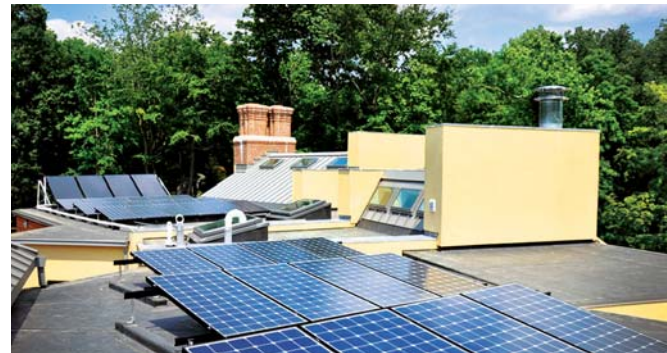
The metal roof features an array of 10-kilowatt solar panels. Excess hot water generated by solar energy is dumped into the geothermal system, pool, and spa. A propane system was added for backup.
